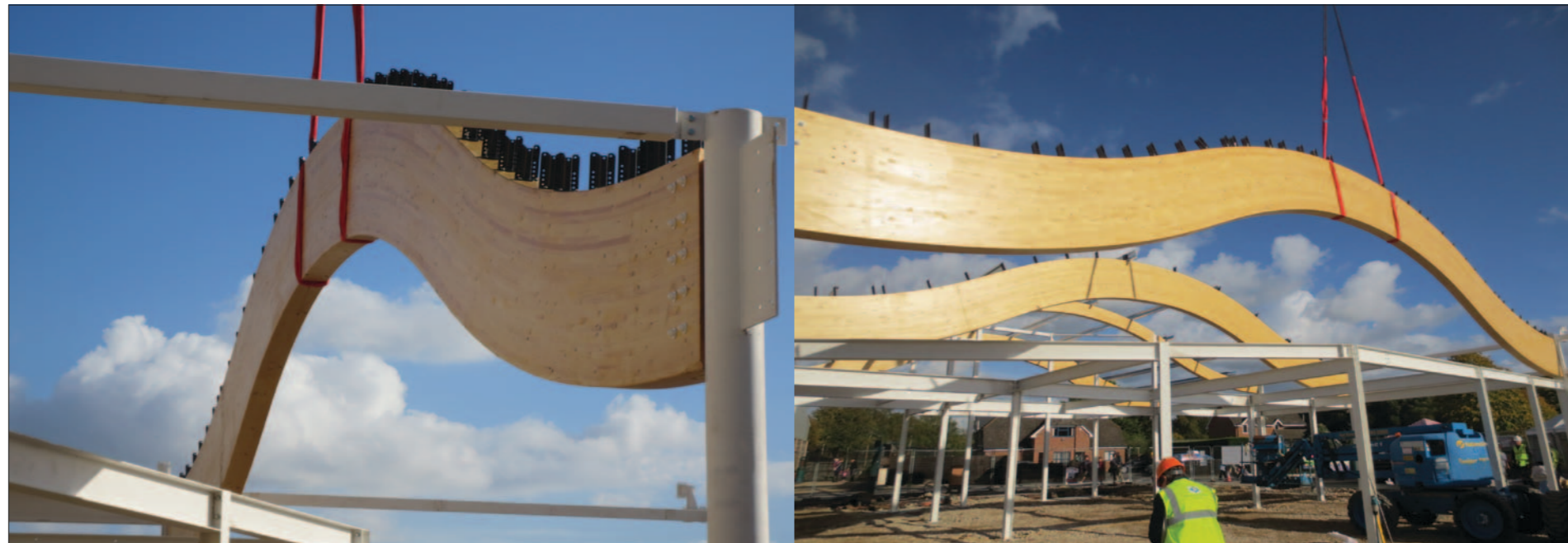
Structural beams made from glulam for the construction of Paultons Park in Romsey, UK
